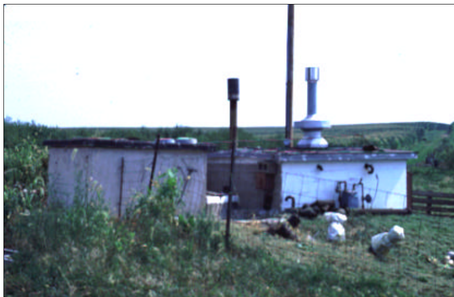
Figure 1. Exterior of anaerobic digester near Mt. Pleasant, Iowa. The digester itself is beneath the control structures in photo. The pipe on the left is used to burn off methane.
