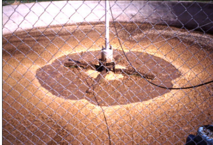
Figure 3. Mechanical aerator in round concrete tank. Air is sucked down vertical pipe into manure liquid.
